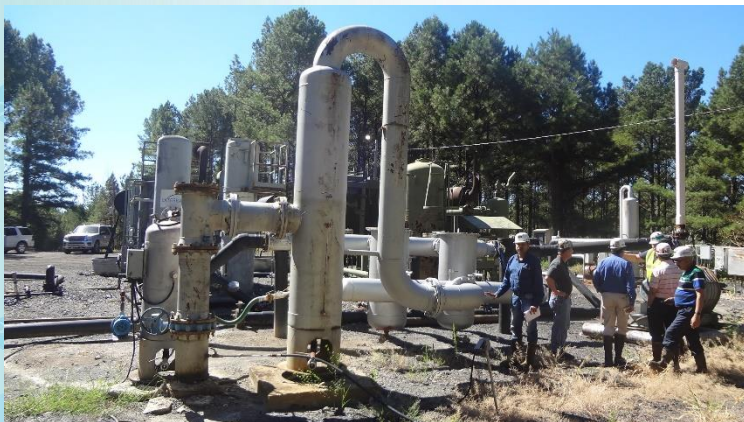
View of GOB well
